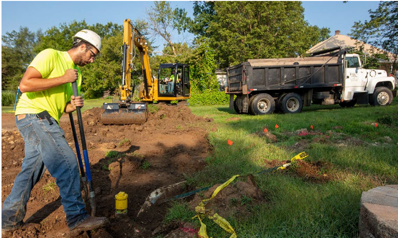
Soil and Land Services remediates yards in St. Francois County. Doe Run continues to make progress on historic mine site remediation projects.
