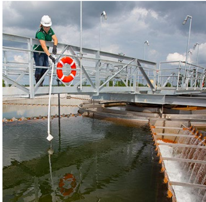
Doe Run’s water treatment plants ensure water that comes in contact with our operations whether at the surface or in our underground mines is treated before it is returned to the environment.
